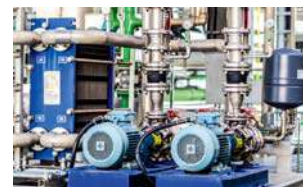
Pump Motor & Gear Box
